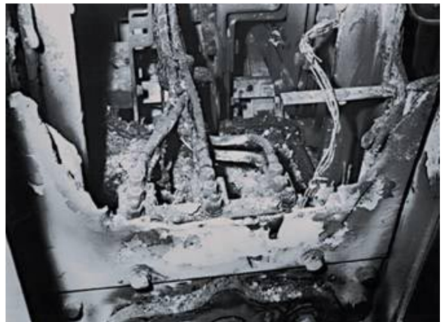
Figure 5: Damage from Arc Fault induced electrical fire (www.arcfault.org)
