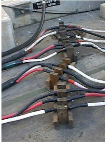
Figure 12-10 A 480-volt shore-cable to ship-cable splice connection in place
