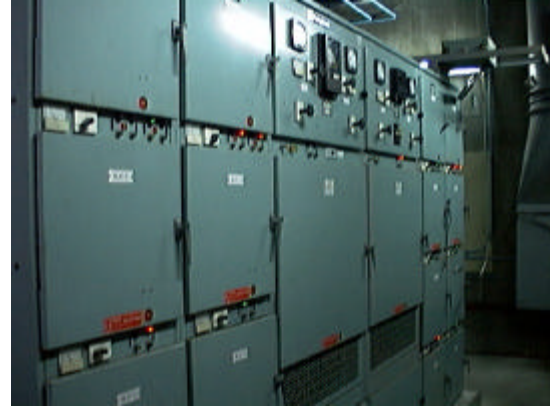
Figure 12-3 A substation inside a pier vault housing
